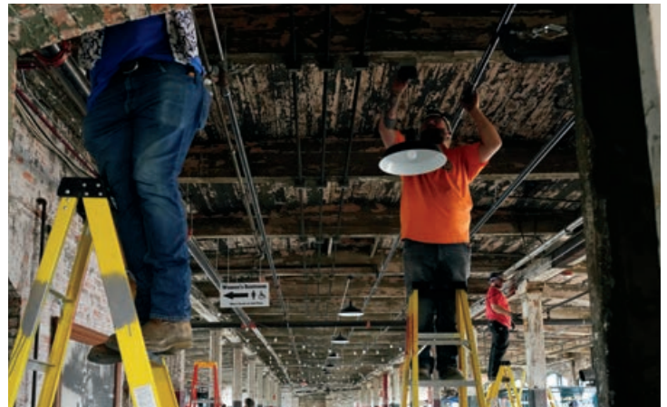
To prevent damage to Piquette’s original wood floors, Motor City Electric used a forest of ladders instead of electric manlifts.
