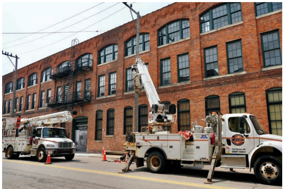
Beaubien Street received new electrical poles and transformers in 2025.
