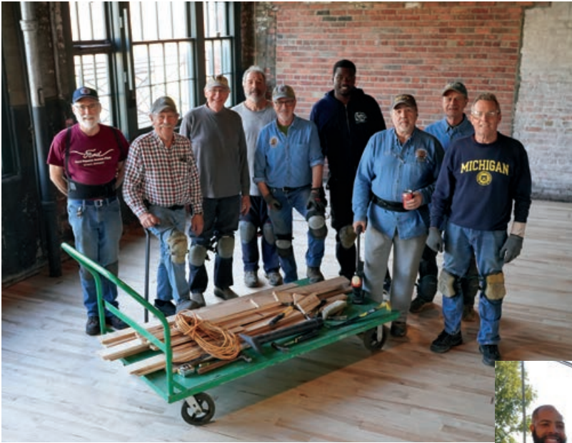
A volunteer team replaced structurally compromised decking boards and flooring in November (L-R): Mark Carpenter, Steve Shotwell, Barry Cogan, Matt Bartolone, Paul Loveridge, Al Collier (museum Building Maintenance Engineer), Joe Mulawa, Jim Valiquette and Doug Nowak.
